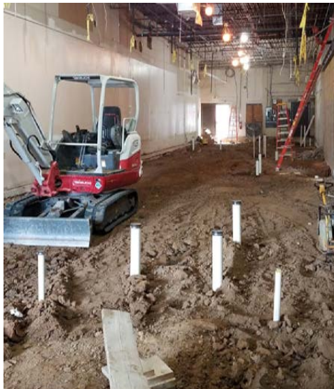
The Willy West expansion started in spring of 2018. The first few months of construction happened in the former Hallmark store space just next door.
